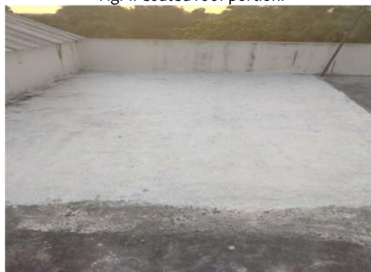
Fig. 1. Coated roof portion.
